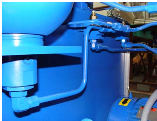
Accumulator lines as delivered with steel line before pressure relief valve
